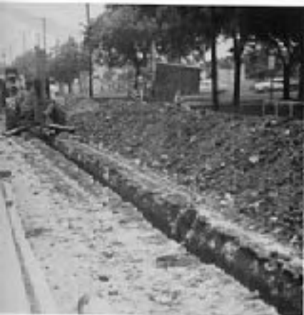
What a new gas line did to our formation site.
